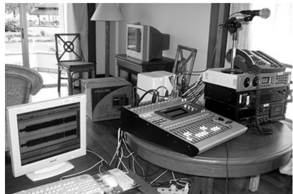
Picture 10 Control Room Sokha Beach Resort Hotel
