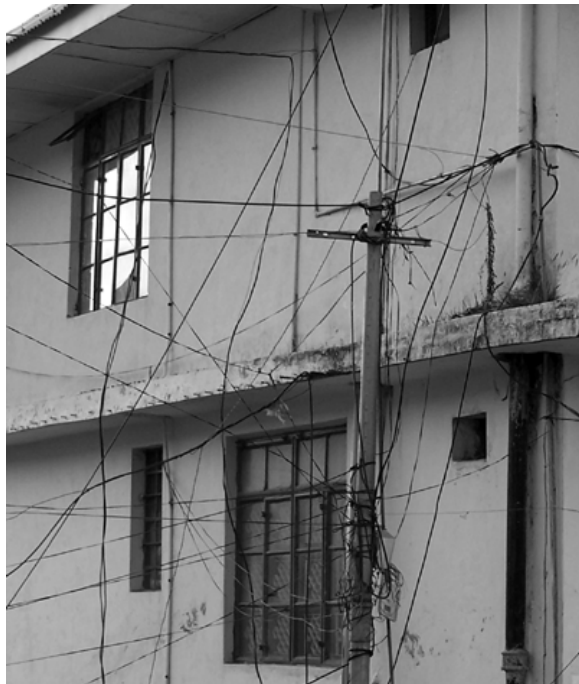
Picture 1 Suspect Piggyback Utility Pole
